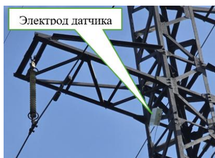
Fig. 2. Geometry of the 3D model of the LK70/110 insulator and its photograph with a capacitive sensor electrode on support No. 66 of the 110 kV "Abdrakhmanovo - Uzlovaya" overhead power line
